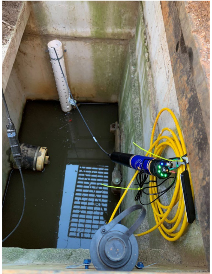
Figure 14: Monitoring equipment installed in outflow structure on site.
